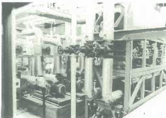
Fig. 3: Services wing plantroom showing one of the two Carrier 300 kW chiller units.
