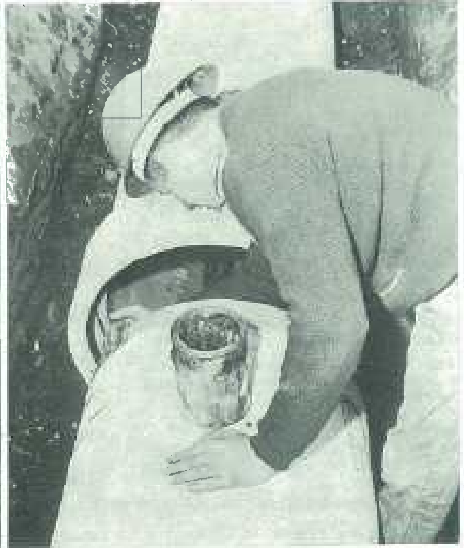
Application of 'Supertite' lubricant to pipe end before insertion into Fibrolite 'Supertite' coupling.
