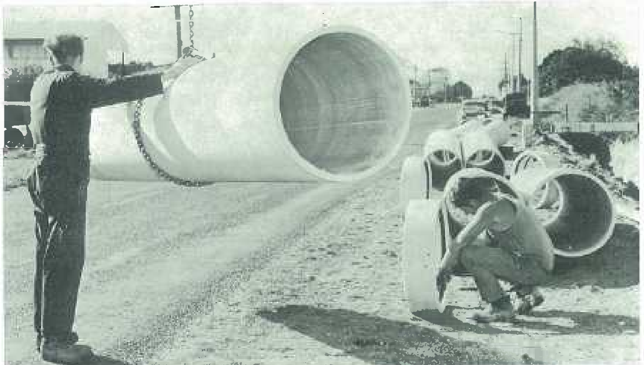
A 24 inch diameter Fibrolite Pipe is ready for laying while rubber rings are placed inside a 'Supertite' coupling. This sewer rising main was designed by the Christchurch Drainage Board. Installation Contractor: George Challey Ltd, Christchurch.
